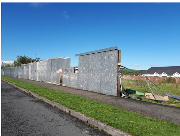
Photo (above): Site/construction hoarding which has rotten and has collapsed and requires follow up with landowner due to health and safety concerns and poor general appearance (UD6).
